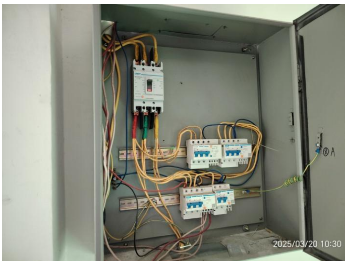
NC 7.13 Electrical control panels missing inner insulation cover and switches not labelled
