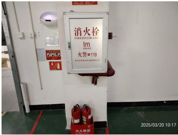
Fire hydrant and extinguishers
