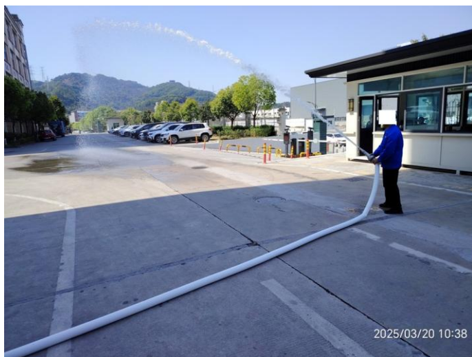
Fire hydrant testing
