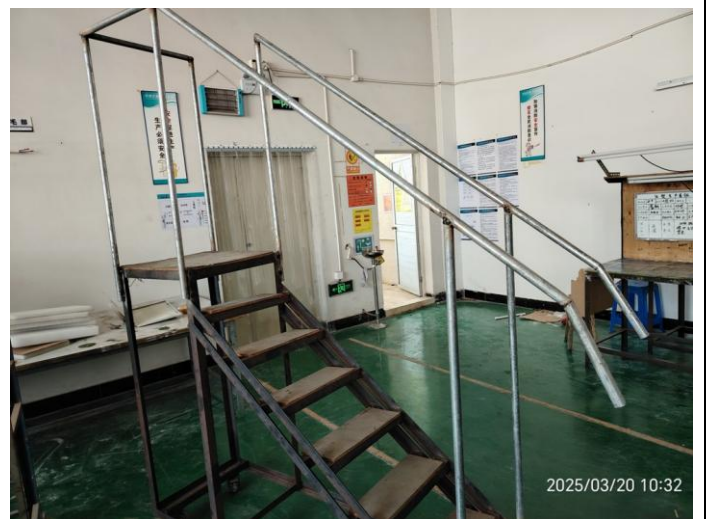
Ladder in injection section installed with handrail
