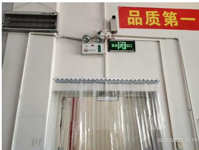
Exit sign and emergency light
