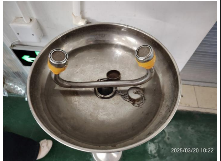
Eye wash station
